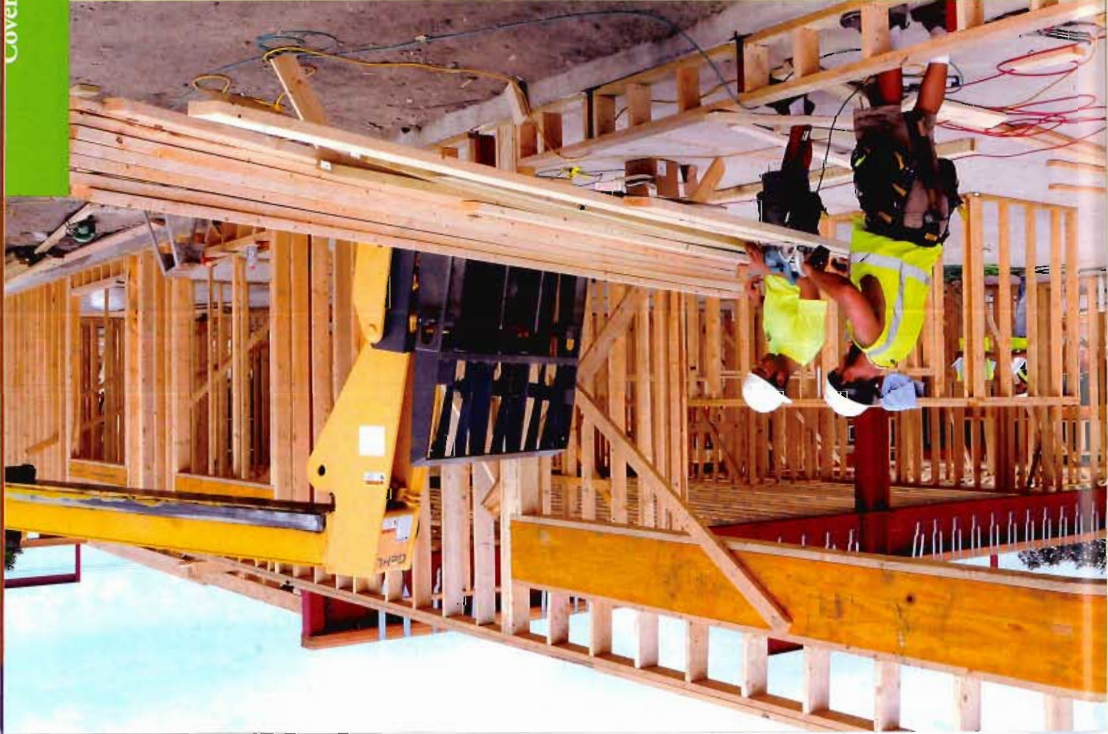
Construction on an office/residential building on the former Marigold site in North Mankato is one of precious few construction projects going on in the region.
